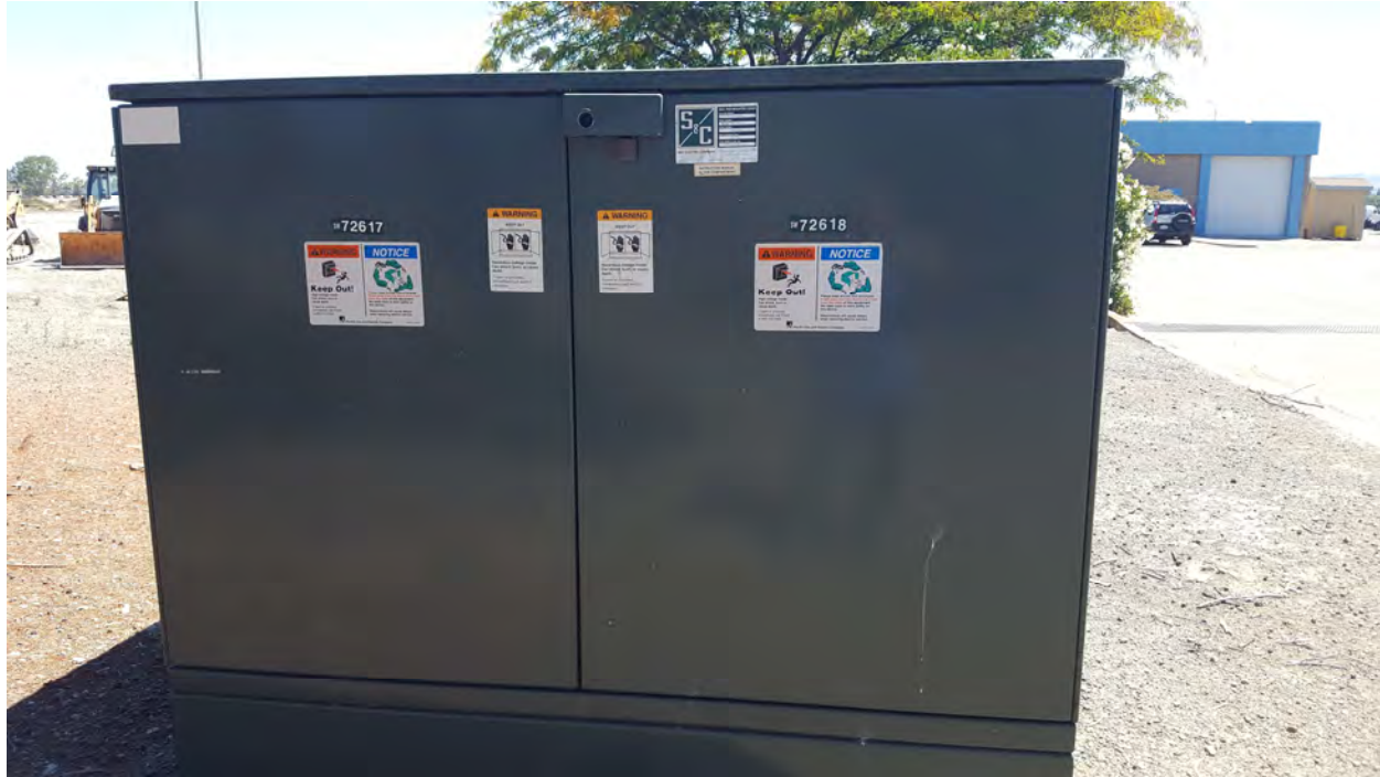
Photo 1 – 21KV Pad-Mounted Switchgear
