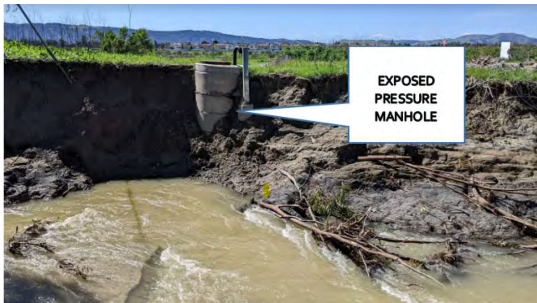
Photo 1.5: Creek Bank Erosion (3/25/2023)
