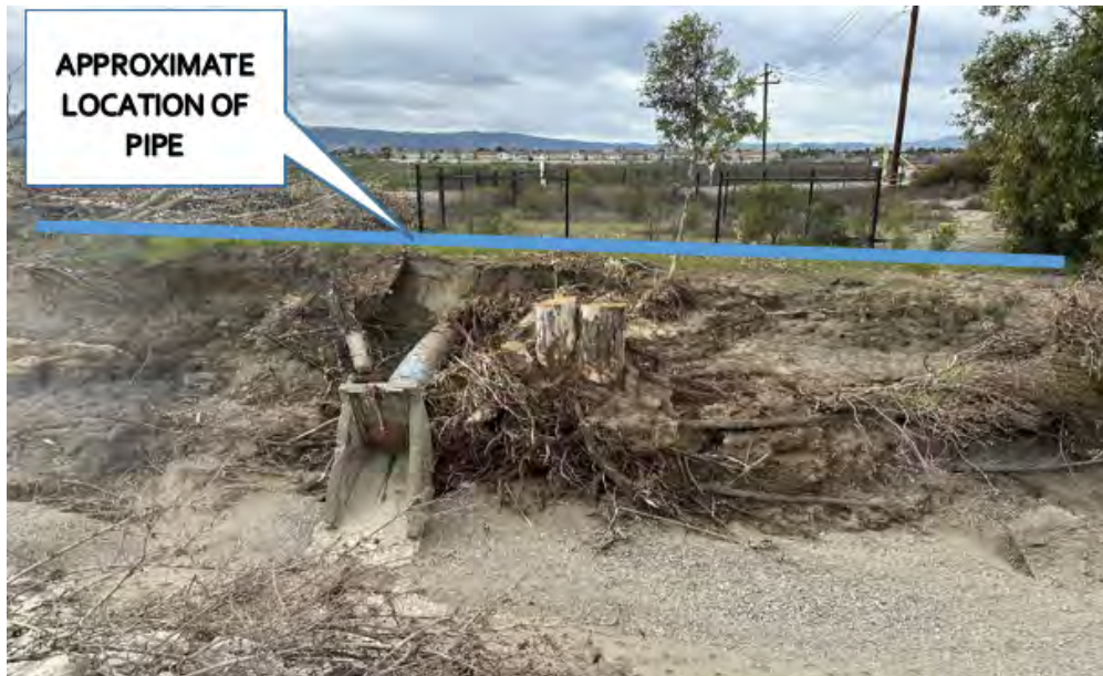
Photo 1.3: Parallel Creek Embankment Risks (2/14/2023)
