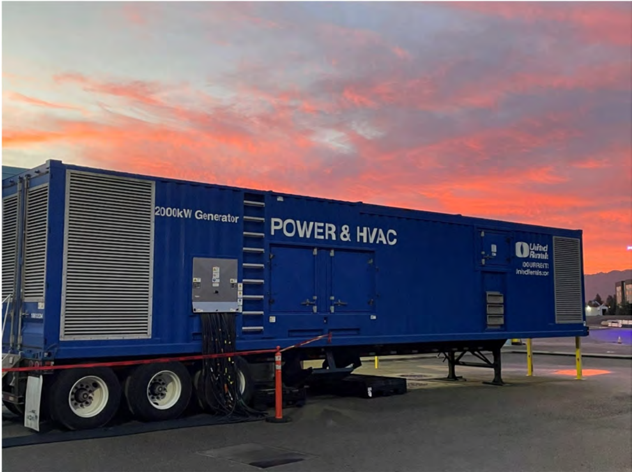
Photo: LAVWMA Rental Emergency Generator, January 12, 2023
