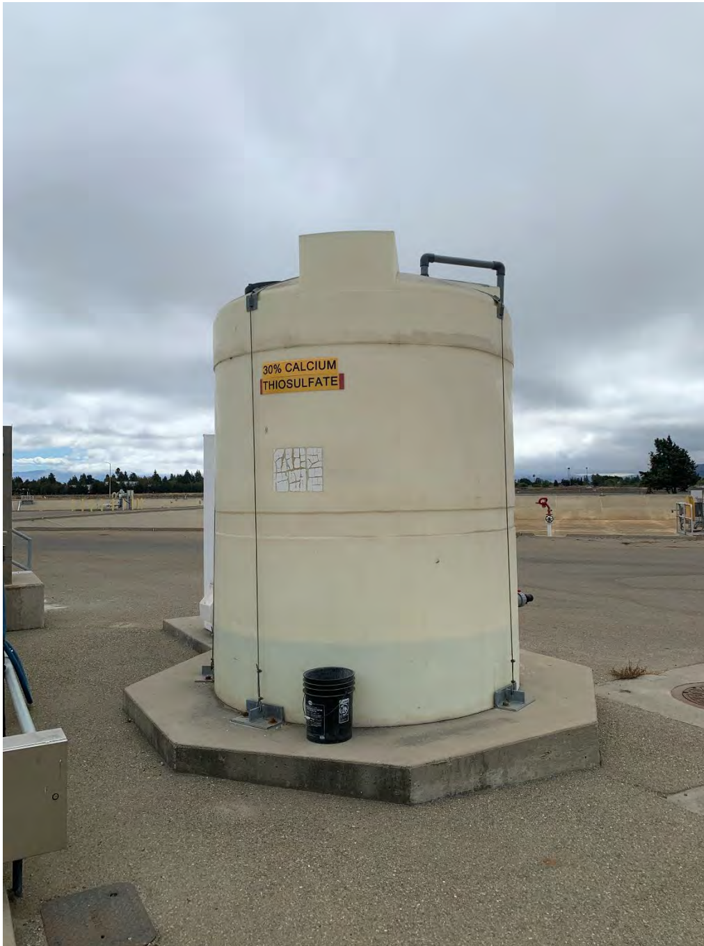
Figure 4. Calcium thiosulfate, for dechlorinating wastewater during wet weather discharges or discharge exercises, was stored within a double-lined container.
