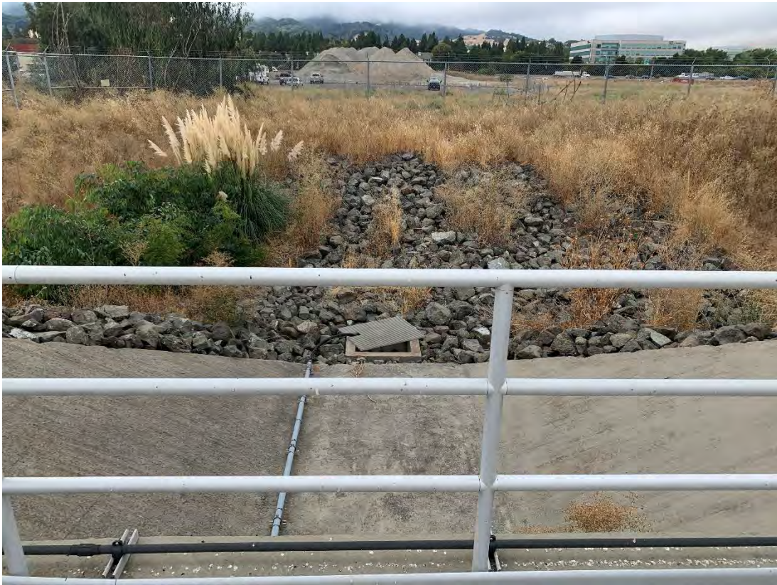
Figure 5. One of LAVWMA's two wet weather outfalls. This one discharges to Alamo Canal.
