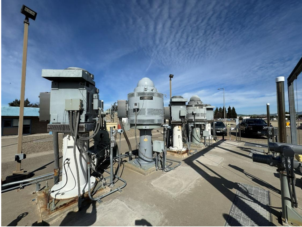
Figure 1. Five out of ten pumps at the LAVWMA pump station.
