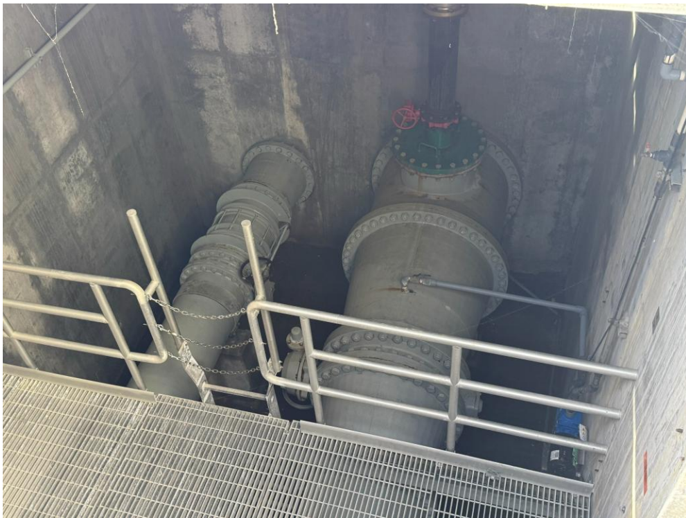
Figure 2. Two pipelines that convey fully treated wastewater from the City of Livermore (left) and DSRSD (right) to the LAVWMA pump station.
