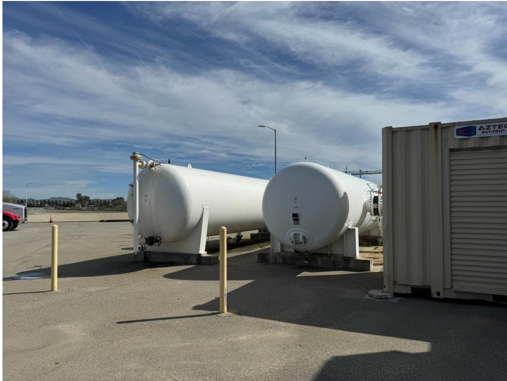
Figure 6. Two surge tanks.
