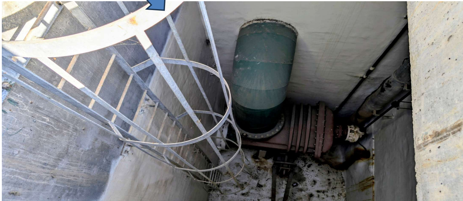
Western Terminus "Gate Valve" valve it successfully isolates LAVWMA from EBDA
